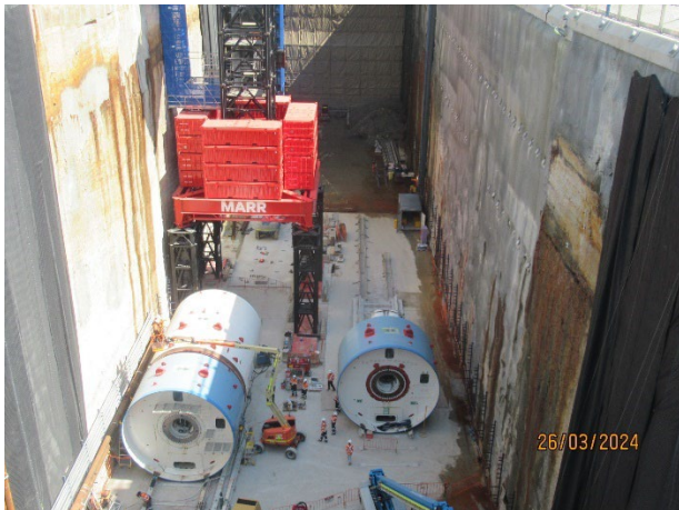
Figure 3.7 The Bays: Tower crane installed in the station box, used to load TBM sections into the station box
