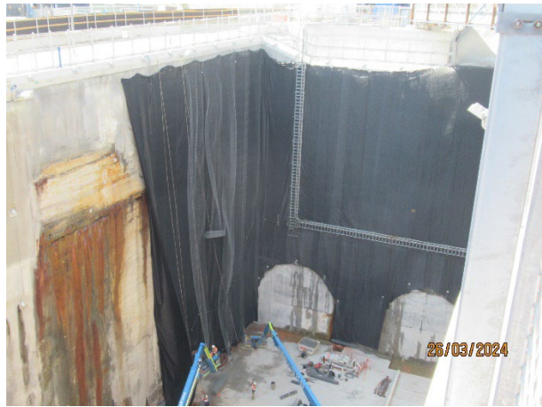
Figure 3.8 The Bays: Steel mesh and fabric mesh placed over the walls of the station box. TBM niches in place.
