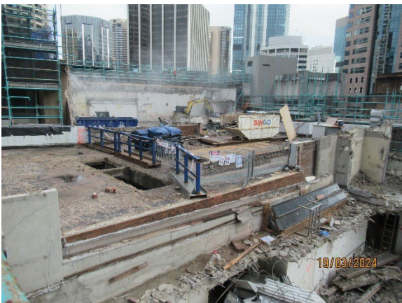
Figure 3.5 Hunter St East: Demolition of the 5m deep beam at the top of 28 O'Connell Street using a rock hammer.
