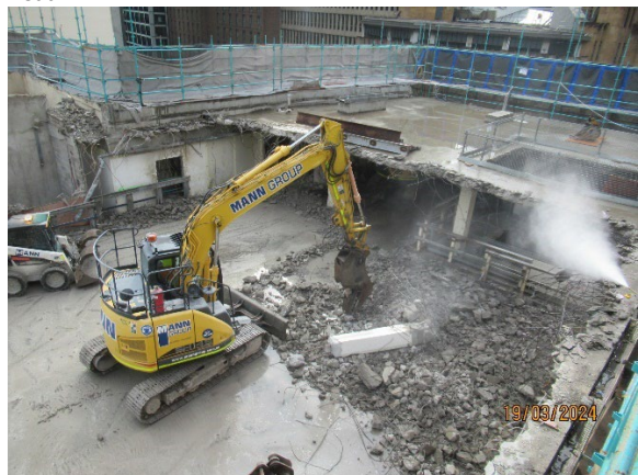
Figure 3.6 Hunter Street East: Use of pulveriser during demolition of 33 Bligh Street Building.
