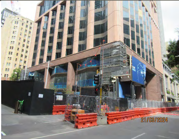
Martin Place South: View from Martin Place. Most of the hoarding removed.
