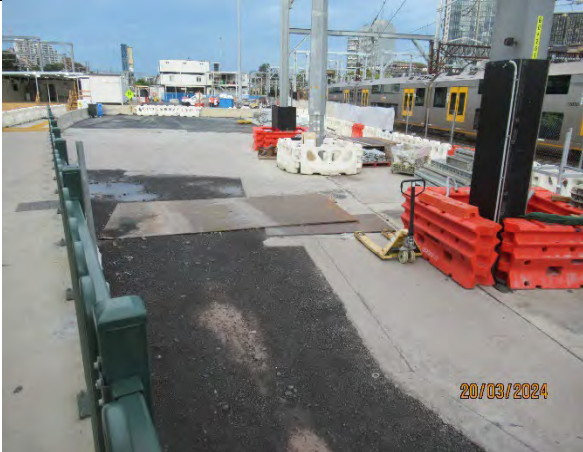
Sydney Yard: View south to where LOR site sheds used to be located – surface has been stabilised with bitumen.
