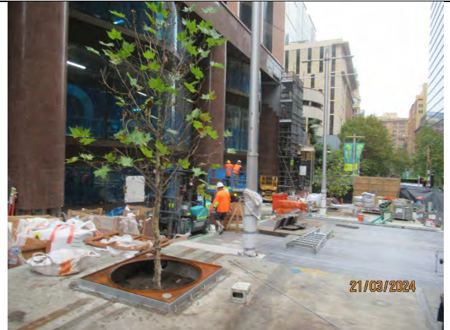
Martin Place: Works in the public area such as waterproofing. Trees planted.
