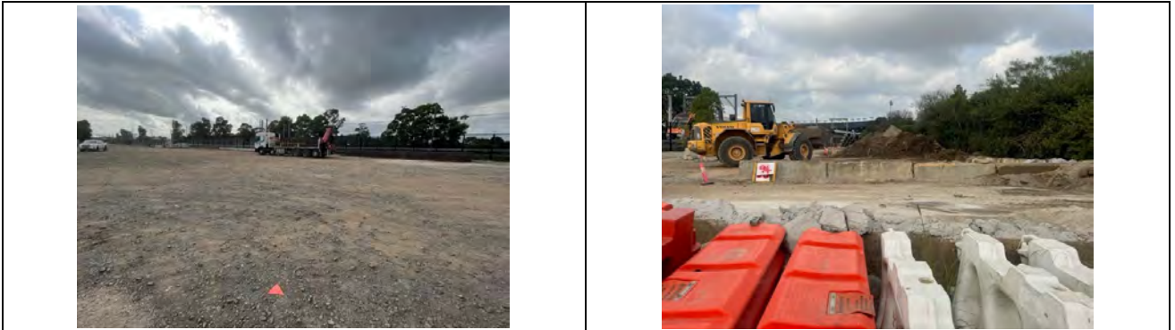
All materials removed from Belmore Triangle in to the approved A17 Ancillary Facility.
