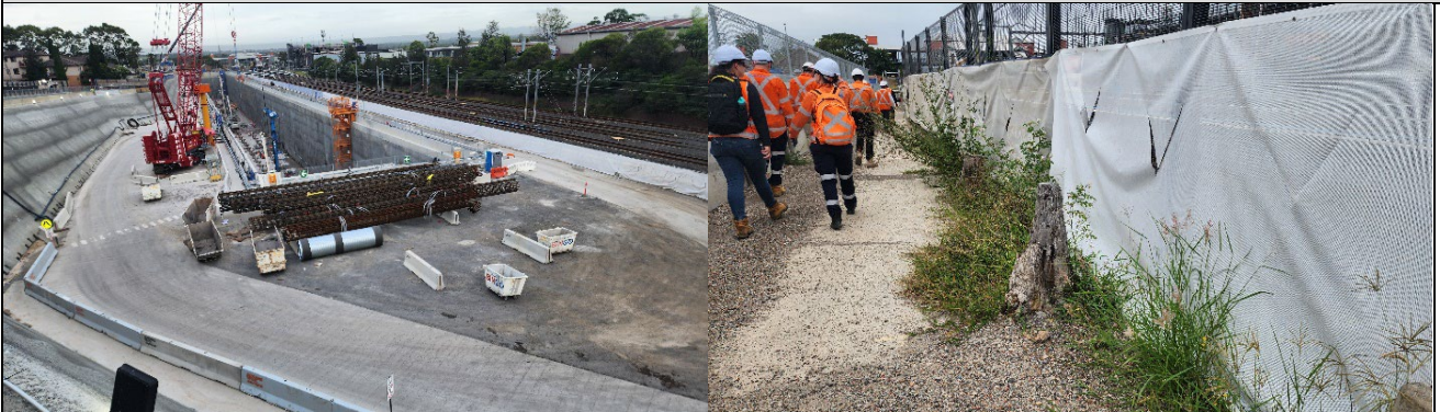
STM – Piling inside of the Box. It was noted that erosion controls were maintained.
