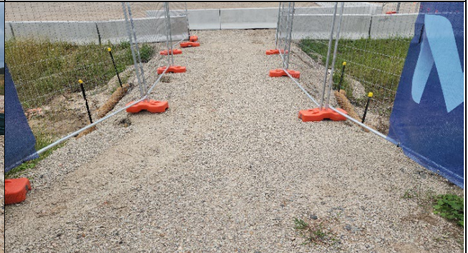
LUD –It was noted that a crossing of the swale required additional erosion and sediment controls. The ER discussed directing flows to minimise scouring..
