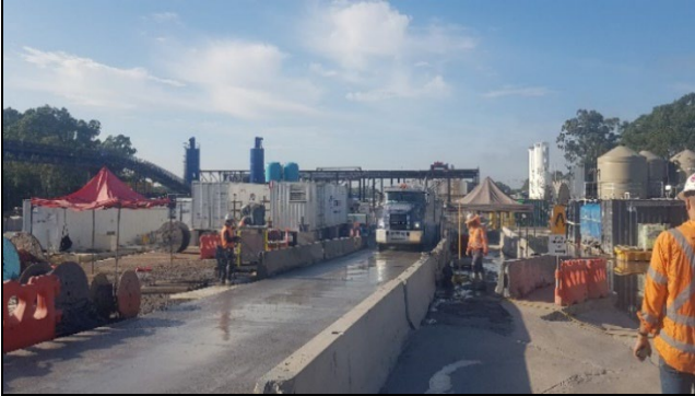
Orchard Hills view south – Internal haul road to exit apron would benefit from more frequent watercart use and sweeping.
