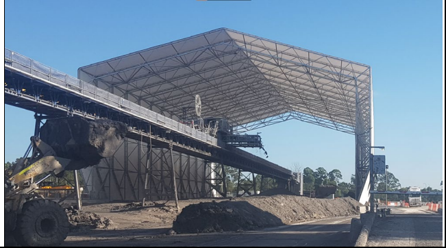
Orchard Hills view north – Tunnel spoil storage area continues to be well managed.
