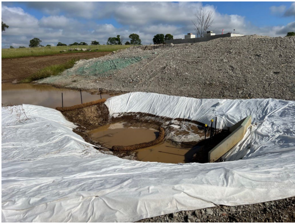
Blaxlands Creek - The turkeys nest arrangement is an example of a control applied where space is constrained
