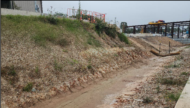
ORH –It was noted that erosion had started to undermine the existing concrete slab. Also noted that weeds had propagated in the area
