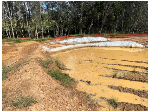
Cosgrove's Creek - ERSED controls on the southern side of Cosgrove's Creek have worked effectively and were in the process of being dewatered
