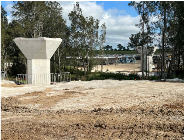
Cosgrove's Creek - Segments are stored in the vicinity of Cosgrove's Creek in preparation for the span across the creek
