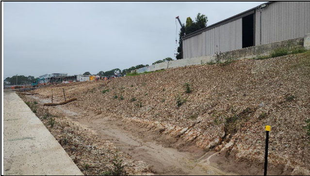
ORH –Reshaping of the batter had commenced; however controls were not installed to minimise erosion
