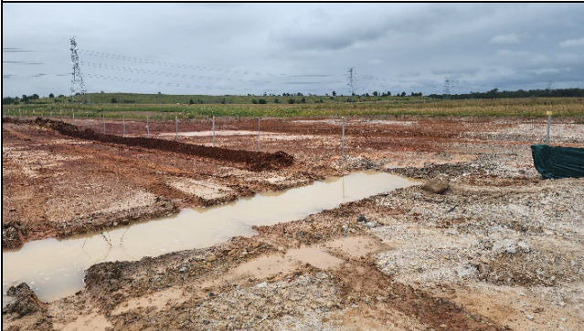
SMF – A drain had been placed across the SMF. It is understood that a retention basin is to be constructed for water reuse onsite.
