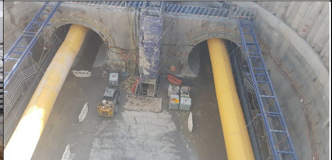
Claremont Meadows shaft view north – Blind rings removed , and pipelines, spoil conveyor system and ventilation system installed.
