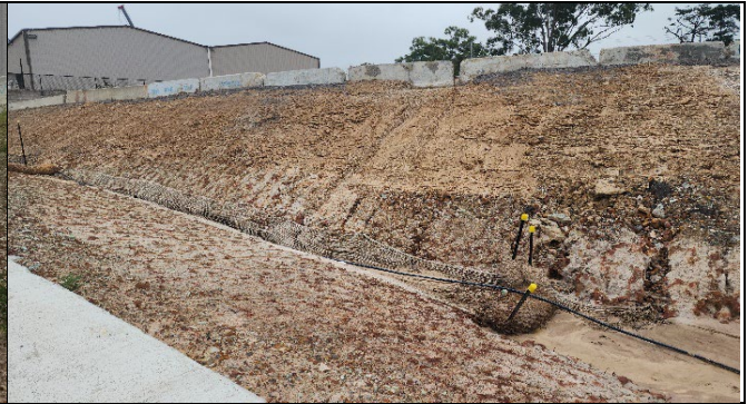
ORH –A section of jute mesh had been placed in the swale; however, no embankment protection was in place
