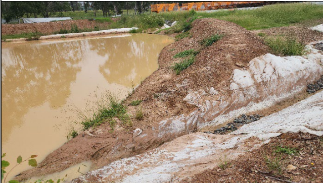
ORH – Geofabric at the sediment basin required re-pining
