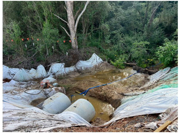
Unnamed tributary - Some debris was deposited downstream of the Unnamed tributary during the recent significant rain event
