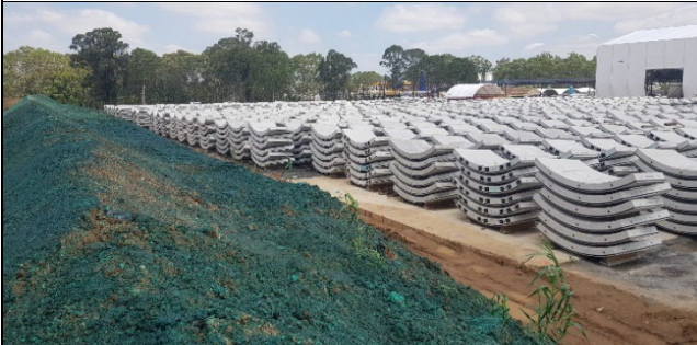
Orchard Hills view south – Stabilisation of spoil stockpile adjacent sediment basin SB8 completed.
