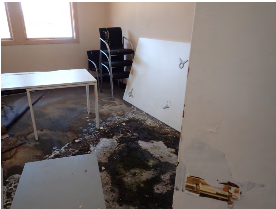
Figure 9 One room has not been used or modified as it had serious mould problems when the TSE team arrived to site.
