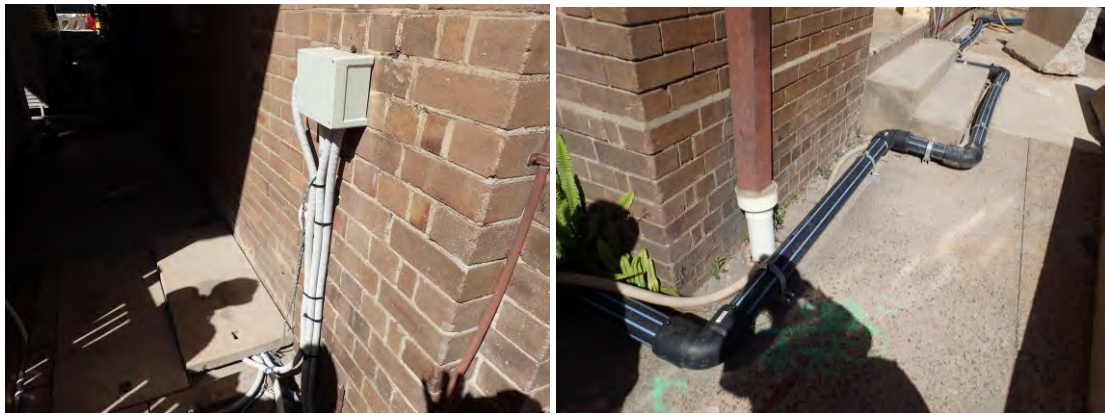
Figure 10 External cabling is fixed to the external wall and will remain in situ (left). Potable water is protected in large diameter pipes which are not fixed to the wall and will be removed (right).
