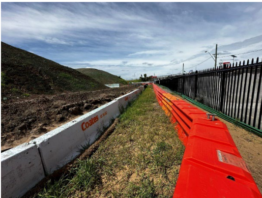
Figure 2.13: Clyde MSF Site – Spoil stockpile controls following rain events
