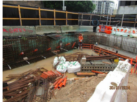
Figure 3.4 Pyrmont West: Construction of retaining wall along Paternoster Row and Pyrmont Bridge Road.
