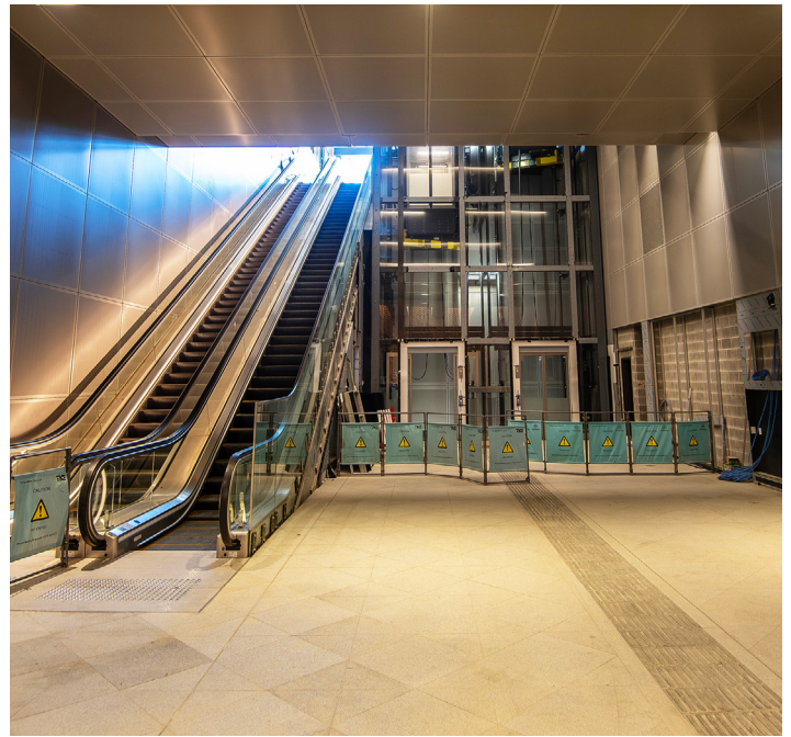
Clarke Street entrance escalators
