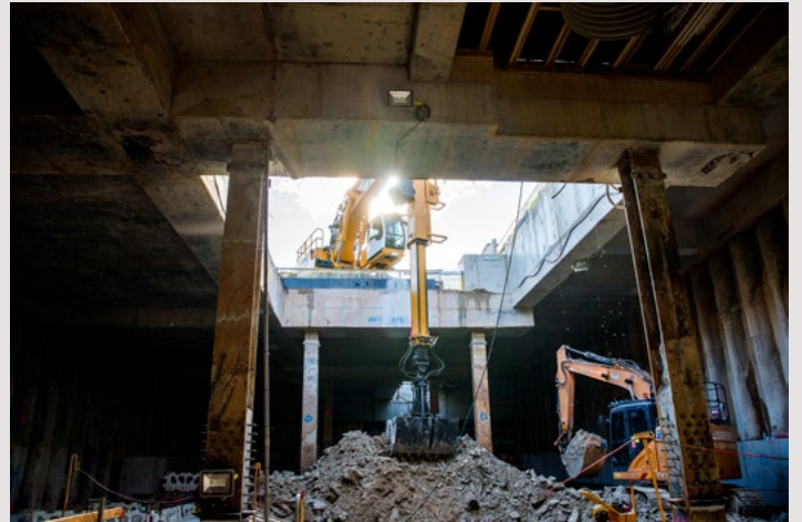
528,000 tonnes of soil was removed during excavation of the metro platforms, enough to fill 88 Olympic swimming pools.
