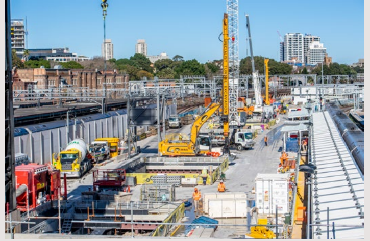
The traffic deck above the new platforms provided access for 24/7 excavation, with rail lines operating either side.
