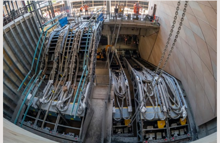
Six escalators were lifted in place through the roof of the building at the Chalmers Street entrance.
