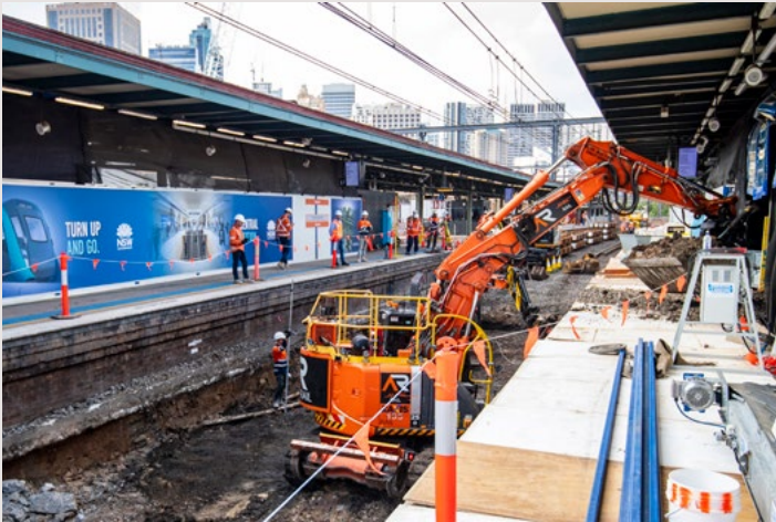
Track work was undertaken on Platforms 16-23 to prepare for the excavation of Central Walk below.
