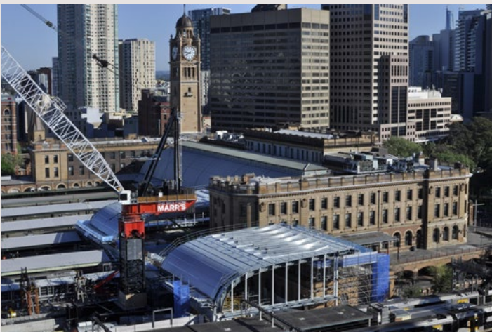
The Northern concourse roof was fabricated off-site and lifted in place one piece at a time during overnight rail shutdowns.
