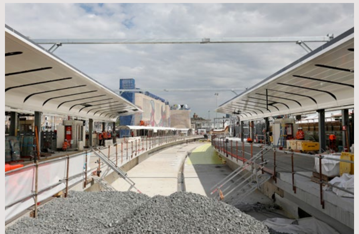
Platforms 13 and 14 were reinstated following the completion of all major works underground.
