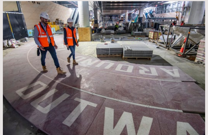
Approximately 1,000 red tiles were installed as part of the public art in the North-South concourse.
