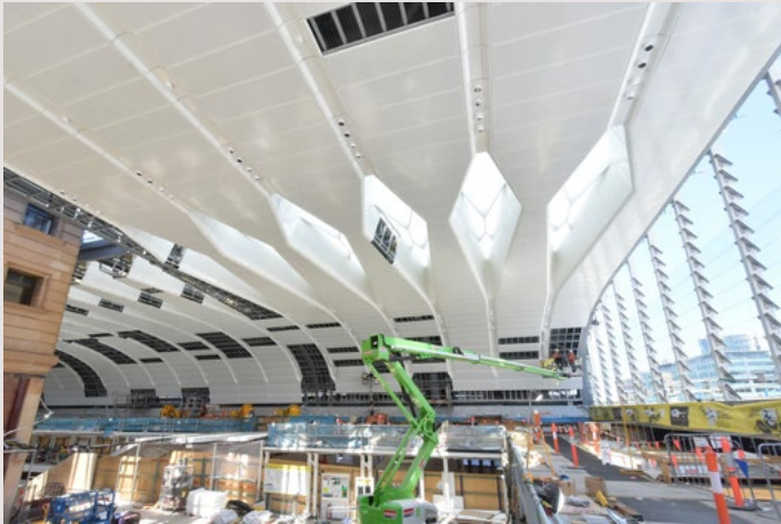
21 diamond shaped skylights provide sunlight through the 80 metres long and 40 metres wide roof.
