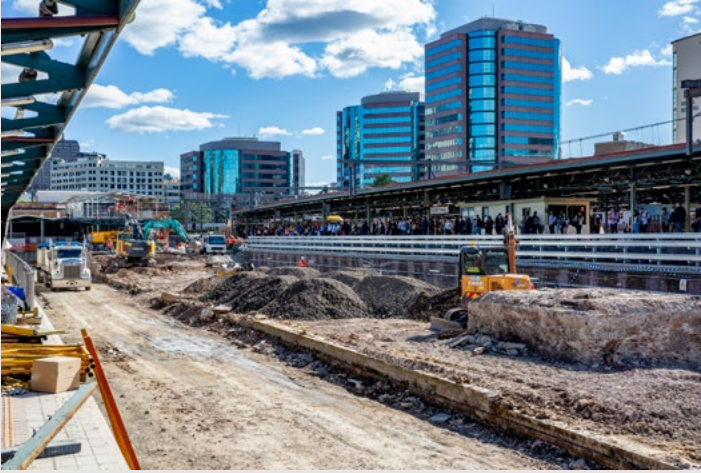
Demolition of Platforms 14 and 15 made way for the excavation of the new metro platforms 27 metres underground.
