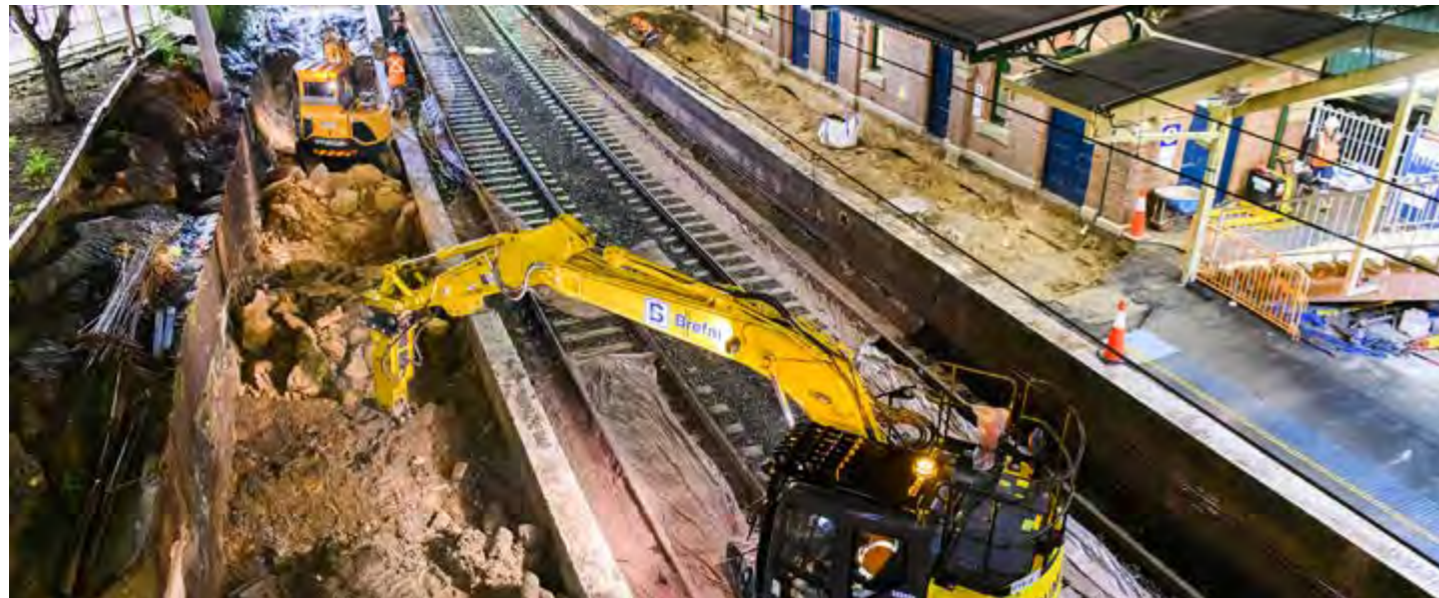
Work to upgrade and convert the tracks and platforms to Sydney Metro standards on the Bankstown Line (Canterbury Station).
