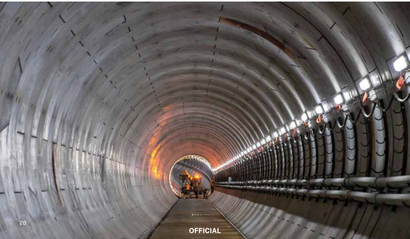
Sydney Metro's under-harbour tunnel construction, part of the Sydney Metro City & Southwest project.
