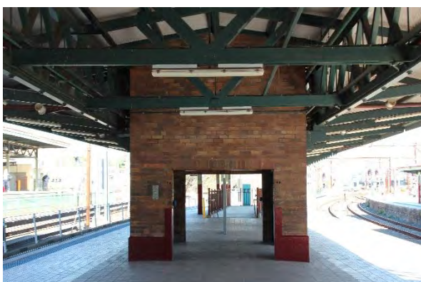
FIGURE 3.35: PLATFORMS 14/15 IN JULY 2018 PRIOR TO DEMOLITION FOR CONSTRUCTION OF THE NEW METRO BOX. THE BRICK STRUCTURE IS A FORMER GOODS LIFT ORIGINALLY USED TO TRANSPORT BAGGAGE FROM THE BAGGAGE TUNNELS BELOW.
