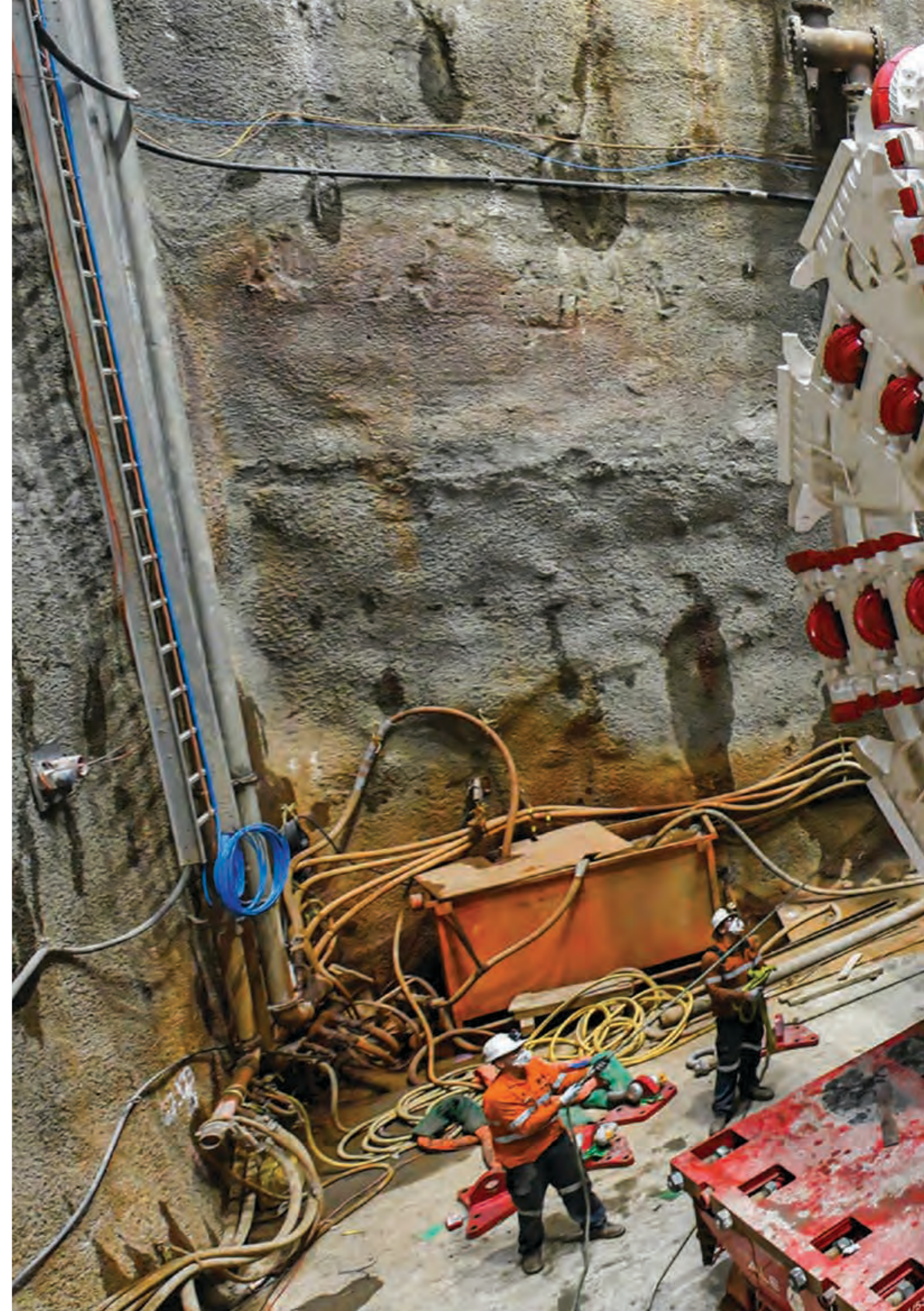
The giant cutter head of TBM 'Kathleen' on the Sydney Metro City & Southwest project.
