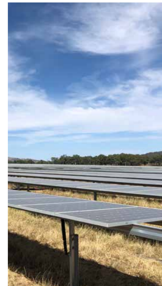
The Beryl solar farm is generating carbon offsets for Sydney Metro Northwest.
