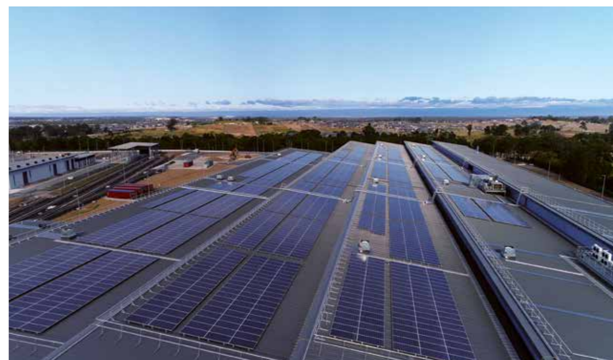
Sydney Metro Trains Facility at Tallawong Road from above, showcasing the 1.1 MW solar array
